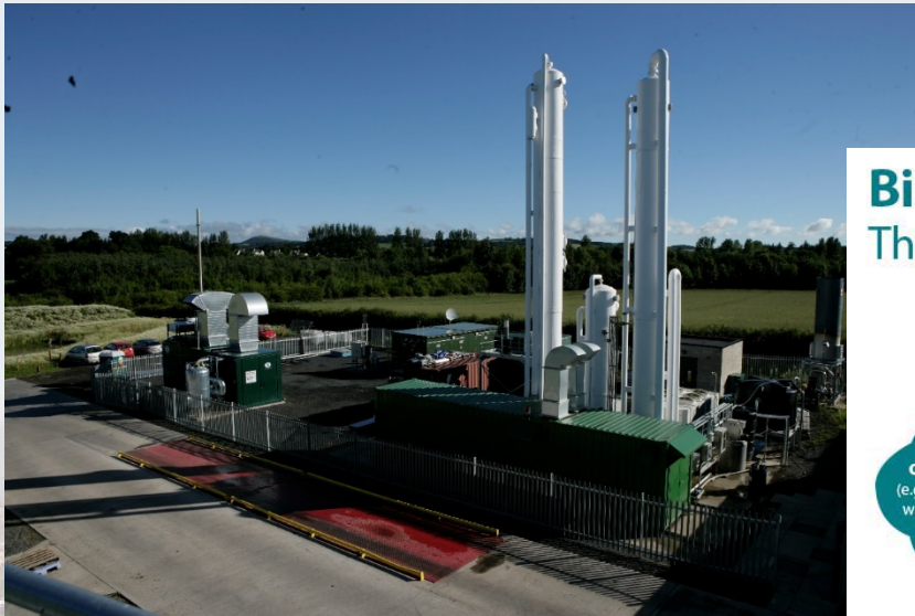
St Boswells Biogas Limited Charlesfield, St Boswells
