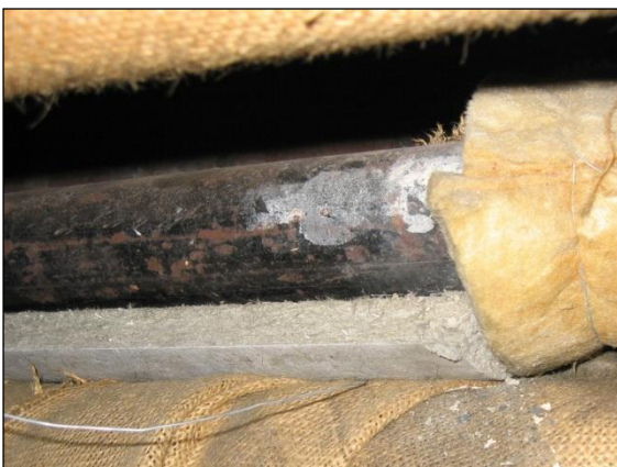
Asbestos pipe insulation
