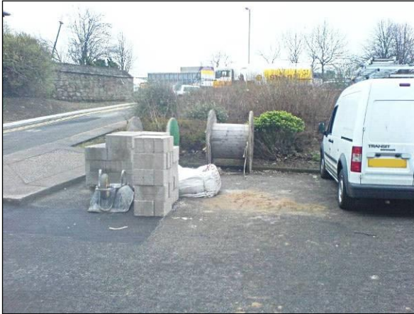
✗ Materials left outside the site compound
