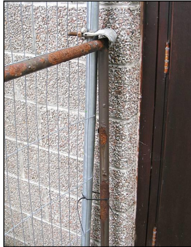
✓ Tie wrap and scaffolding clamp
