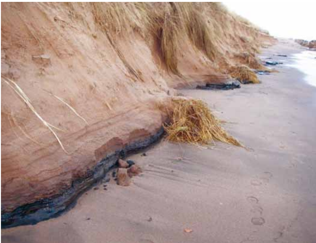
Figure 5.37 Leachates are clearly visible at the toe of the foredunes (Hastings, E. 2008)
