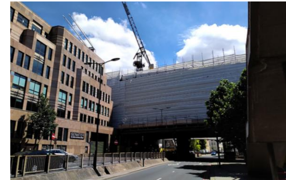
Buildings located over public highway, London, UK, showing the presence and protection interfaces.
