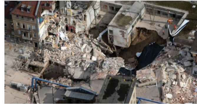
Collapse of multiple buildings resulting from excavation collapse, due to metro construction, Cologne, Germany. Source: National Research Council, 2013.
