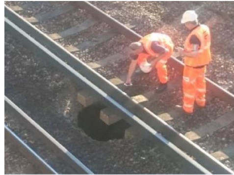
Sewer collapse, under railway, Forest Hill, UK, 2016. Source: BBC, 2016.
